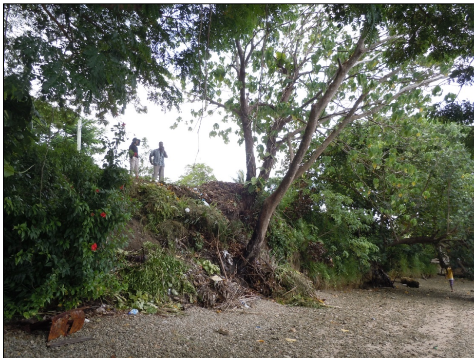
Figure 43 Erosion near Coral Quay
