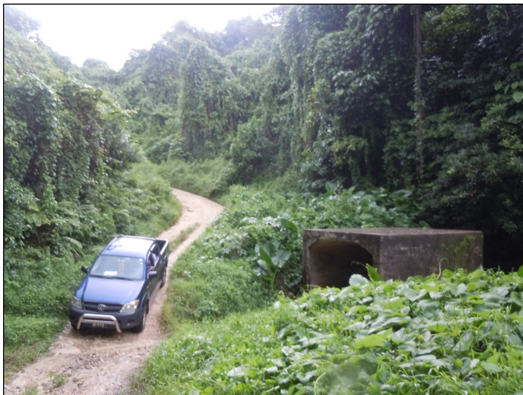
Figure 49 Culvert Carried away by water
