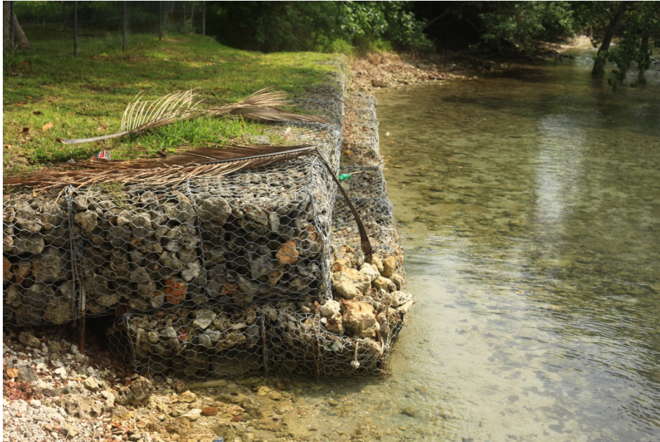
Figure 26 Gabions deteriorating due to lack of Geotextile membrane
