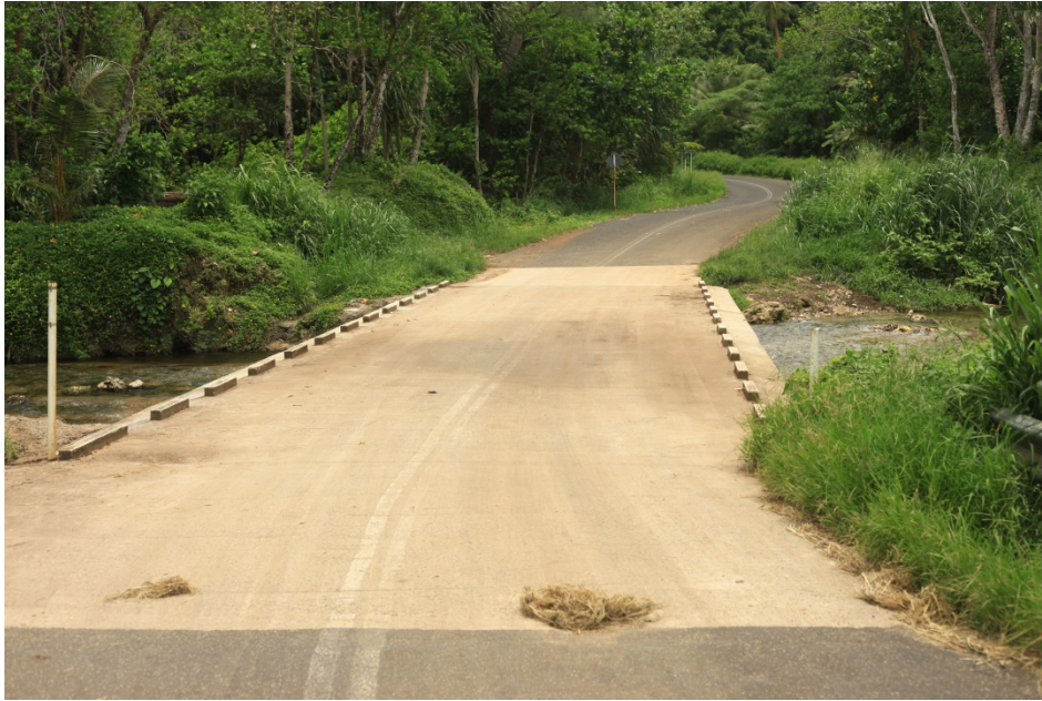
Figure 20 Vented Road crossing with concrete safety blocks
