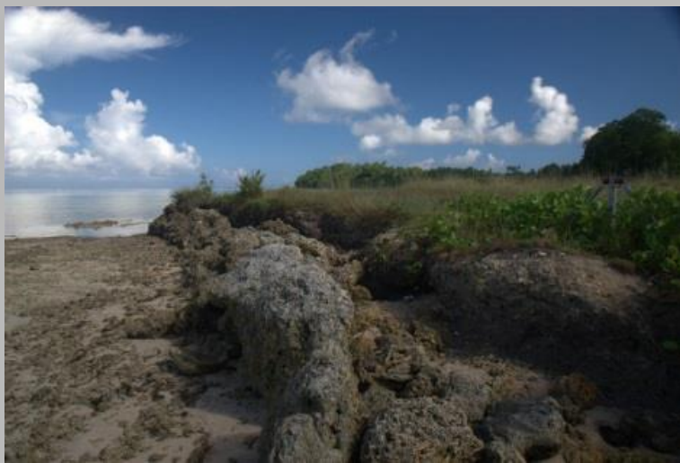
Plate 5: Northern end of Taro airstrip at low tide. Note active erosion behind existing coastal protection rip rap.
