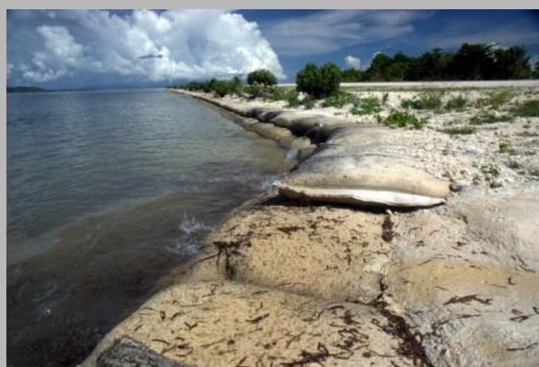
Plate 9: Contextual example of newly installed coastal protection - geotextile bags filled with sand at the Nusatupe airstrip.
