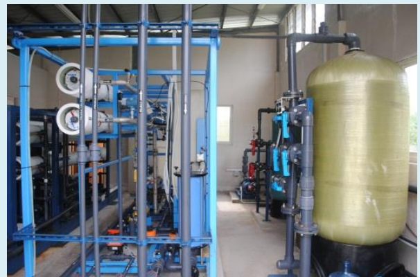
A desalination plant at the Public Works Department
