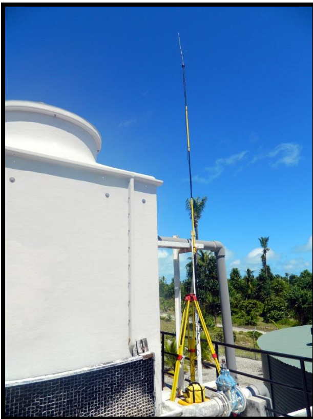
Figure 8. To increase radio coverage, the radio antenna was mounted on top of the Public Utilities water tower.
