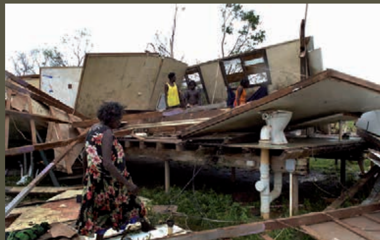
Damage from Cyclone Monica, 2006. Image: Newspix
