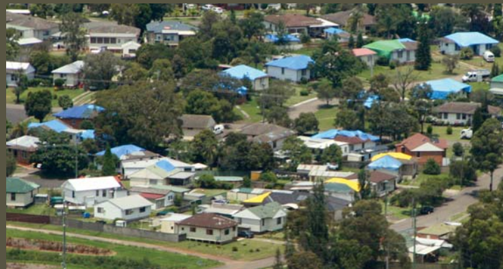
Tarpaulins cover hailstorm damaged roofs, Blacktown, NSW, December 2007. Image: NSW State Emergency Service.
