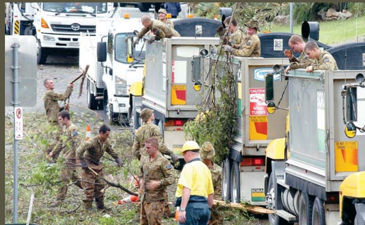
Clearing storm damage in The Gap, Brisbane, 2008. Image: Commonwealth of Australia/Graham McBean.
