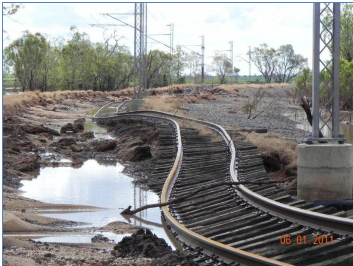
Figure 1 Rail damage January 2011 in Comet Region, (photo courtesy of Gladstone Regional Council).
