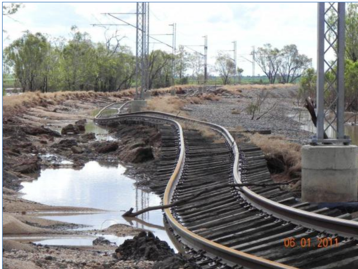
Figure 1 Rail damage January 2011 in Comet Region, (photo courtesy of Gladstone Regional Council).
